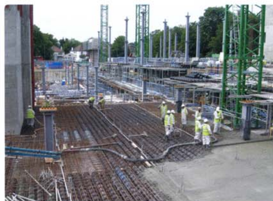
Figures 3 and 4 right and overleaf: Using Hanson's Cobiax system, the whole frame for the new Tesco Stores development in Orpington went up in just 40 weeks – almost twice as fast as solid slabs.
