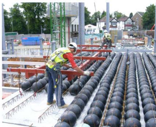
Figure 2 right: Hanson's Cobiax precast concrete panels are used to create large spans without the need for supporting beams and columns.
